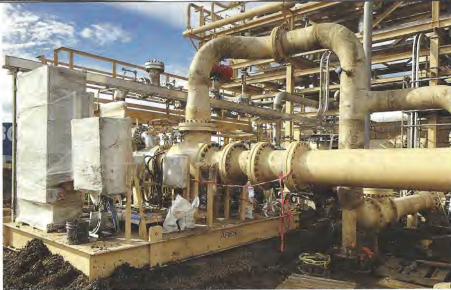
The commissioning process for the first ARES Active Magnetic Bearing Turboexpander-Compressor saw cold and wet conditions.
